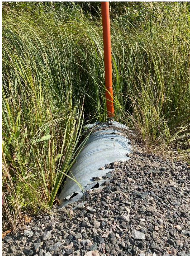
Figure 3: Culvert Damage due to Insufficient Cover (McDonald Rd.)
