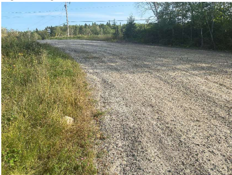
Figure 2: Organic Obstructed Ditch (Carlton Road)
