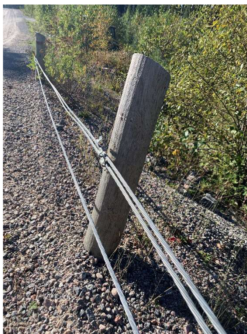
Figure 11: Loose 3CGR Cables (North Marston Dr.)
