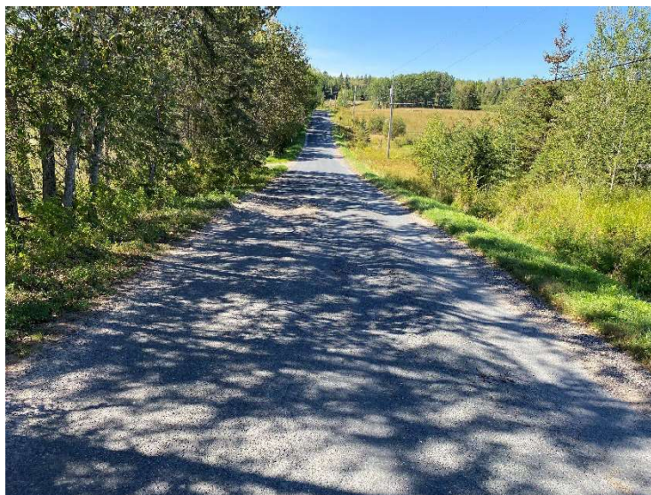
Figure 4: Rutting in Surface Treatment (James Rd.)
