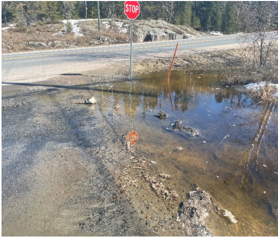
Frozen Culvert Barsky Crescent
