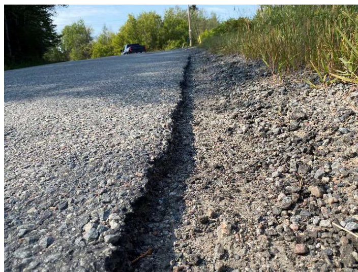
Figure 10: Low Shoulder (Anderson Rd.)
